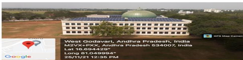
SOLAR PLANT ON CENTRAL LIBRARY
